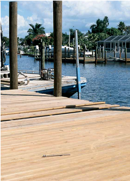
Elevated Service / Severe
