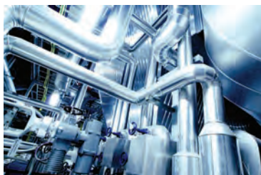
Typical high-corrosive environment — central utility plants.
